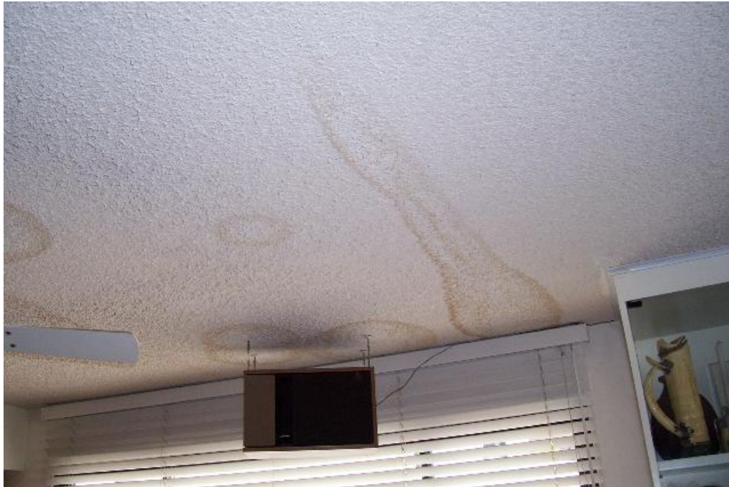
PF 01.070 PF 01- 070.jpg Unit C dining room: Ceiling stains surrounding ceiling fan and above speaker. The floor is concrete.
