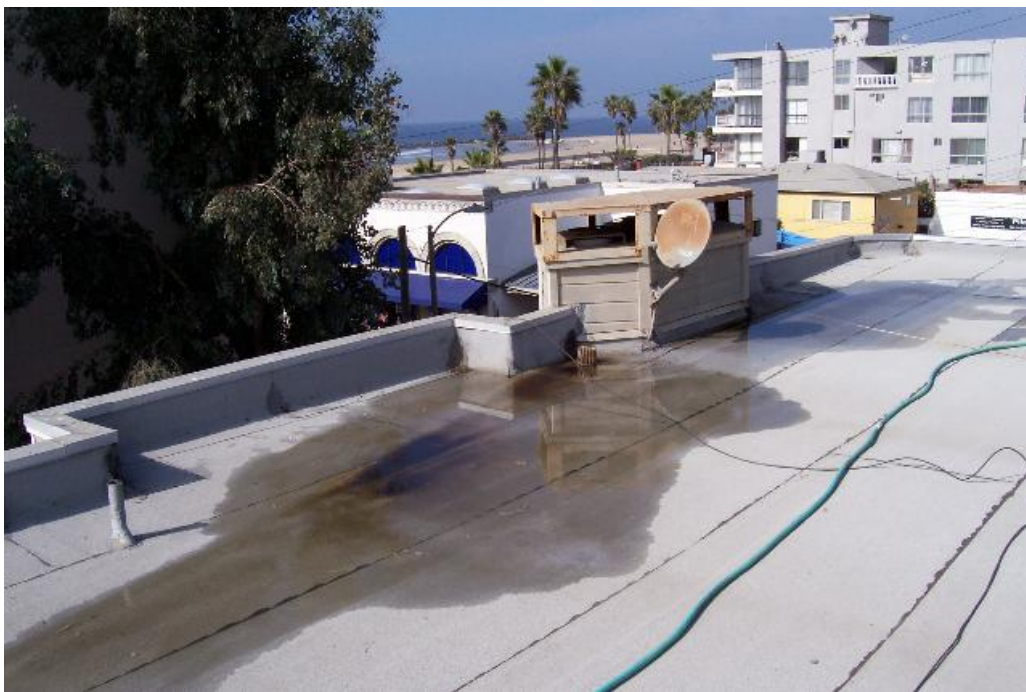
PF 01.135 PF 01- 135.jpg Roof test A: water is ponding around drain at right elevation near chimney.
