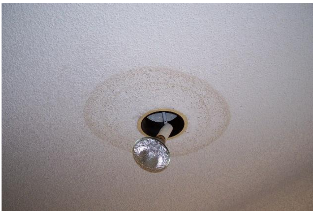
PF 01.097 PF 01- 097.jpg Unit C bedroom #2: ceiling stain at can light in center of room, at back and front.
