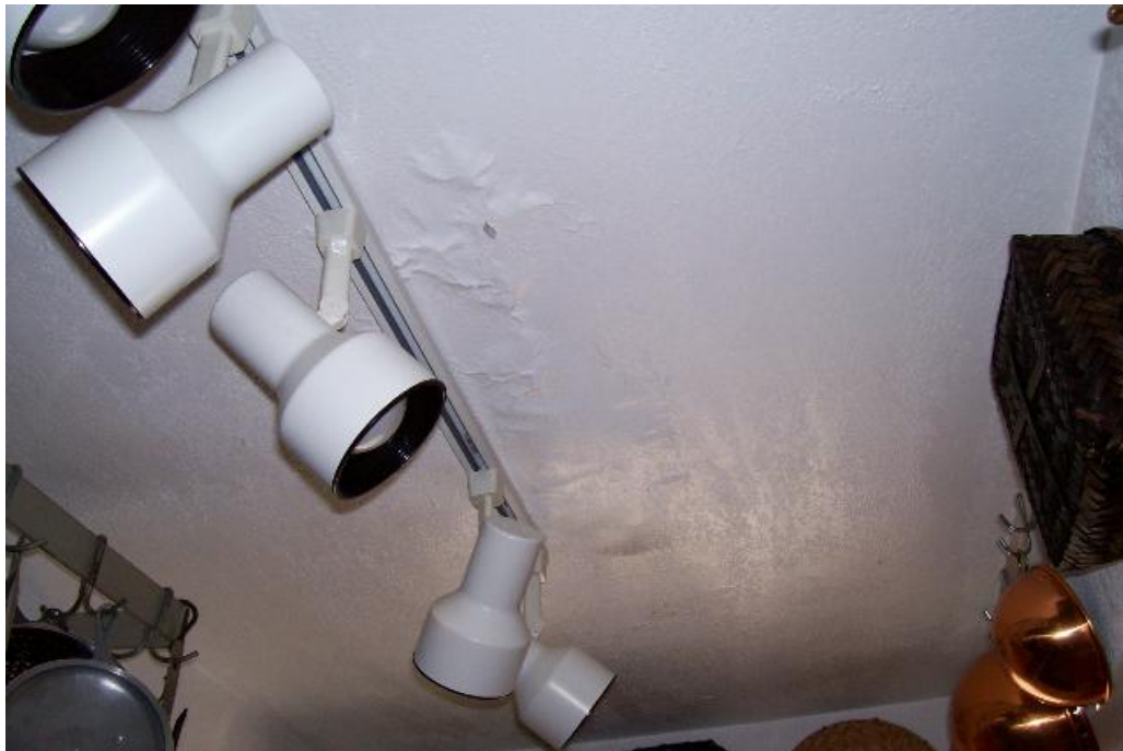
PF 01.083 PF 01- 083.jpg Unit C kitchen: Ceiling damage.
